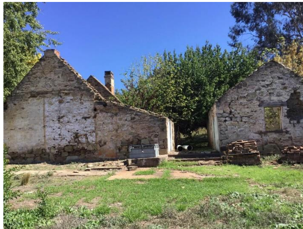
This photo is taken of the right side of the home showing clearly the separate kitchen and wash-room at the rear (right in this photo). There is a tree growing inside one of the rear two rooms of the main home.
